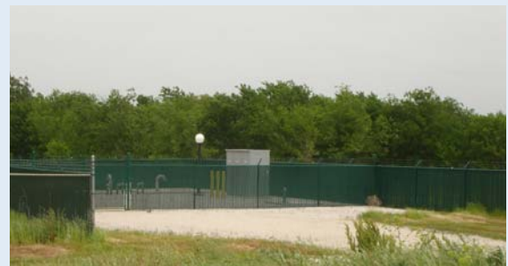
West Side Lift Station
